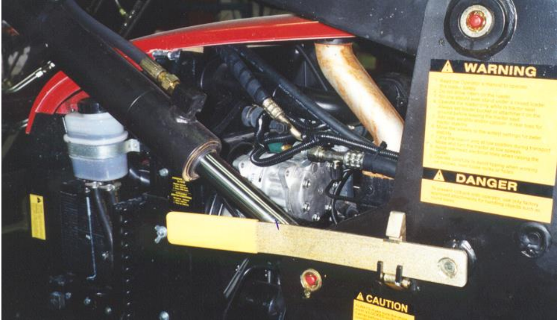
Hoses and fittings at compressor.
